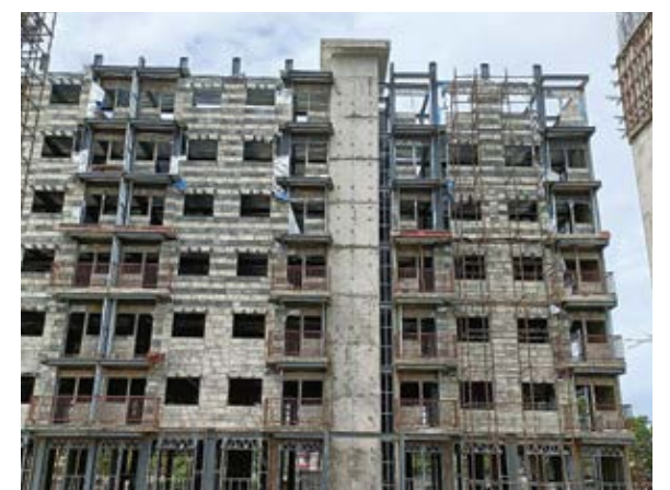
Fig.16: Placement of Precast Concrete Panels filled with Light Weight Concrete in LGS frames
