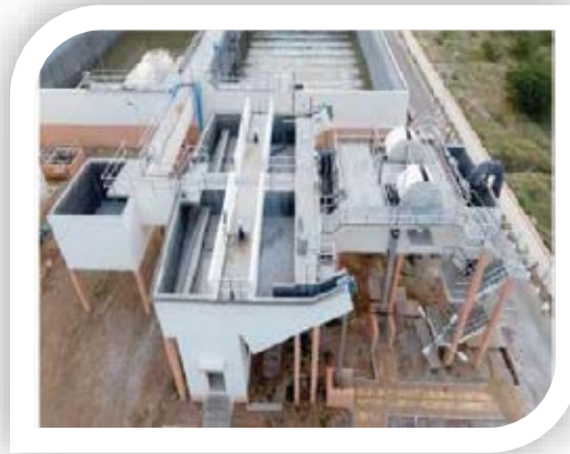
Sewage Treatment Plant in Davanagere
